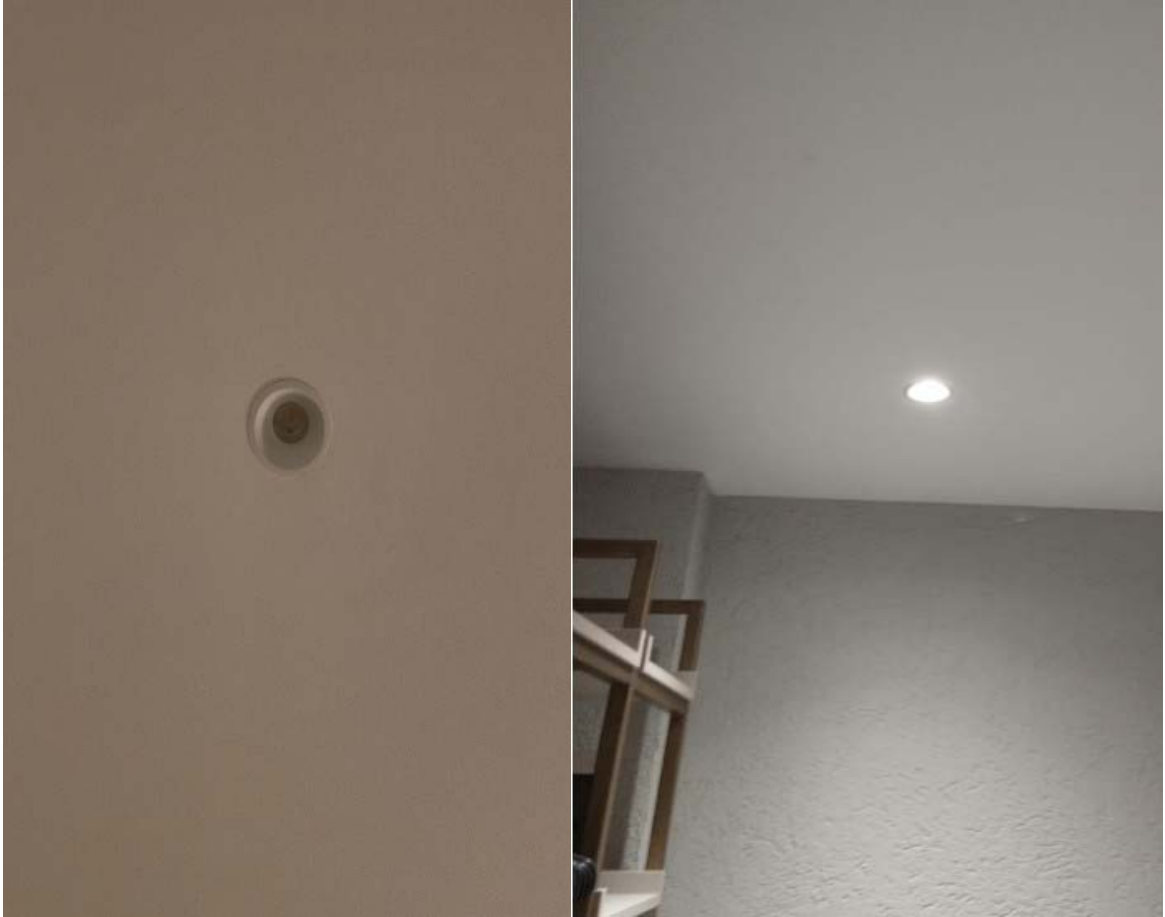
Room lighting is also provided with LED lights.
